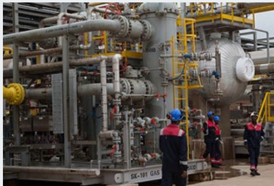
Atuabo gas plant in Ghana 54
